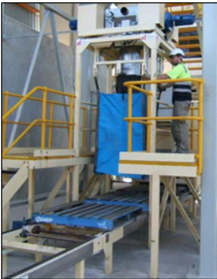
Figure 24-36 - Automated Filling System
